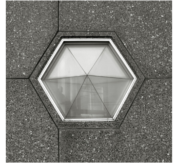
27. Hexagon window in the gravel concrete ground level underneath the Shell tower in 2012.
